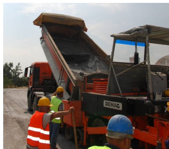
Figure 3. Fresh concrete stuck on the truck due to delay in transportation
