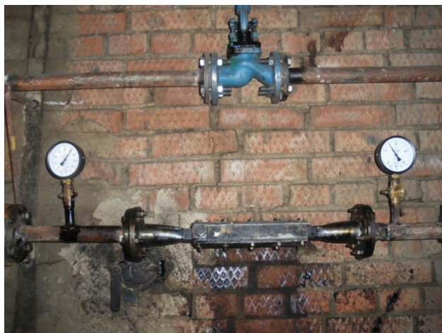
Fig.4. General view of the unit for water-oil emulsion preparation for combustion in the boiler furnace.
