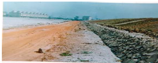
Fig. 5. Dyke constructed with fly ash at Korba Thermal Power Station, Madhya Pradesh
