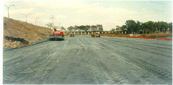
Fig. 1. Nizammuddin bridge approach road embankment at New Delhi (in flood zone of river Yamuna)
