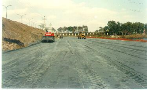
Fig.2. Nizammuddin bridge approach road embankment at New Delhi (in flood zone of river Yamuna)
