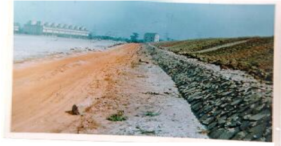
Fig.10. Dyke constructed with fly ash at Korba Thermal Power Station, Madhya Pradesh
