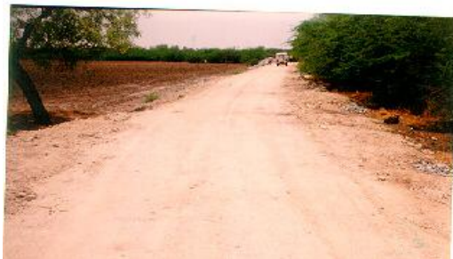
Fig.3. Raichur- Arsnagi road, via Yadlapur in Raichur distt. Of Karnataka. The fly ash road (in unmetaled condition) has performed well for last 7 years
