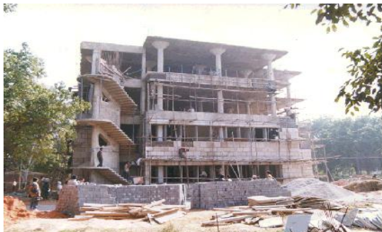
Fig.4. Four storey building constructed using flyash bricks at Indian Institute of Technology, New Delhi
