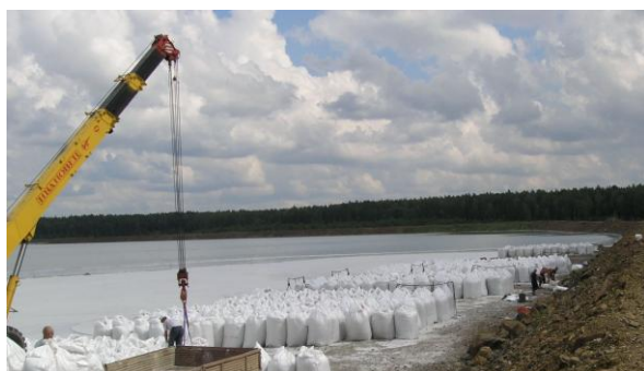
Fig. 3. Loading of fly light fly ash fraction gathered from ash disposal lagoon with the use of technology of Omega Minerals Group
