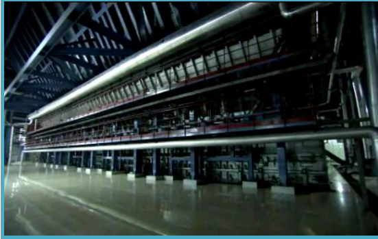
Fig. 9. The first air-cooled dry bottom ash handling system applied under 2x1000 MW boiler in the world.
