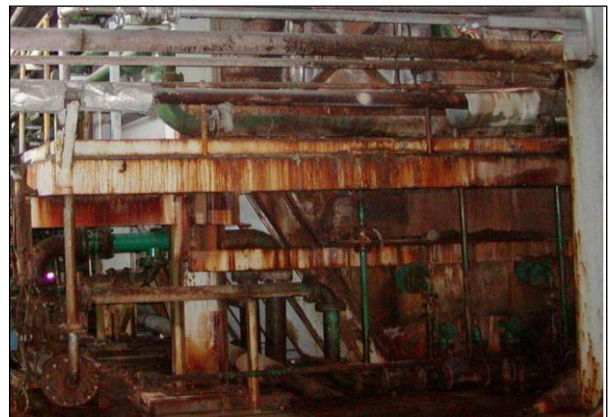
Fig. 7. The Corrosion of Traditional Wet Bottom Ash Handling System.
