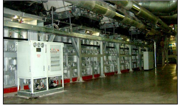
Fig. 8. The Clean Working Environment of 4x600 MW Air-cooled Dry Bottom Ash Handling System.
